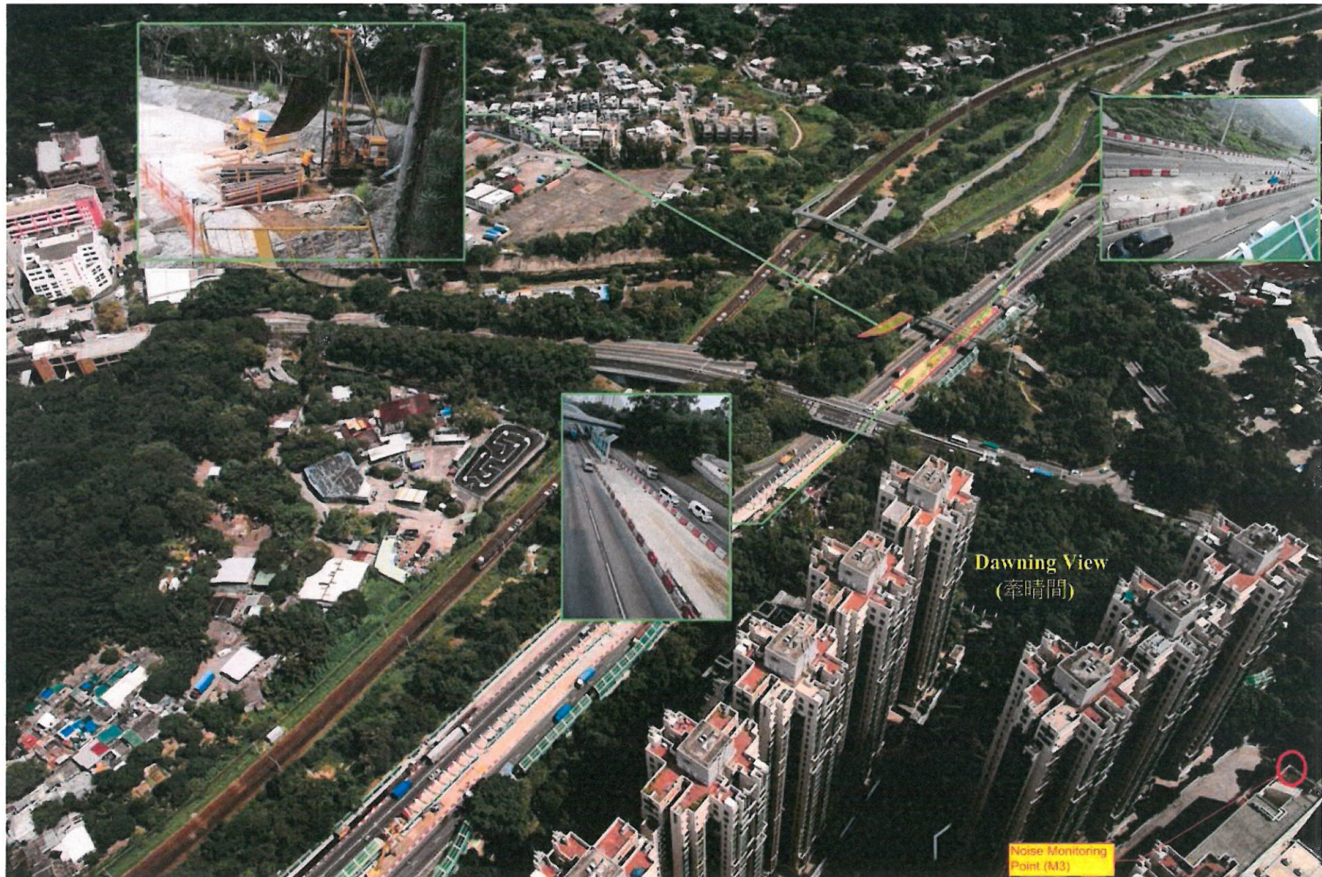
Figure 1 - The location of construction works on 18 June 2014 near the noise monitoring location M3: Wo Hop Shek Pedestrian and Cyclist Bridge
