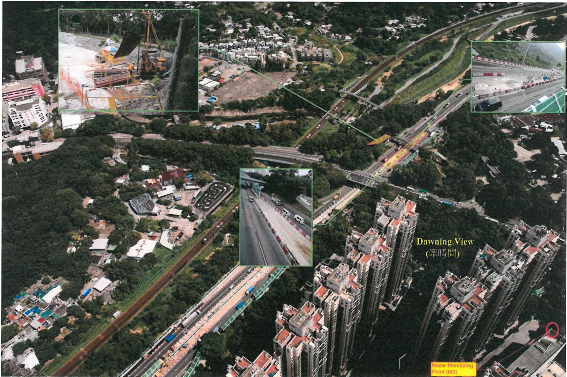
Figure 1 - The location of construction works on 18 June 2014 near the noise monitoring location M3: Wo Hop Shek Pedestrian and Cyclist Bridge
