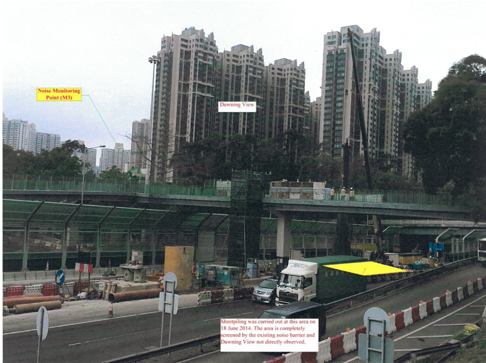
Figure 2 – The works area screened by existing noise barriers and residential buildings at Dawning View
