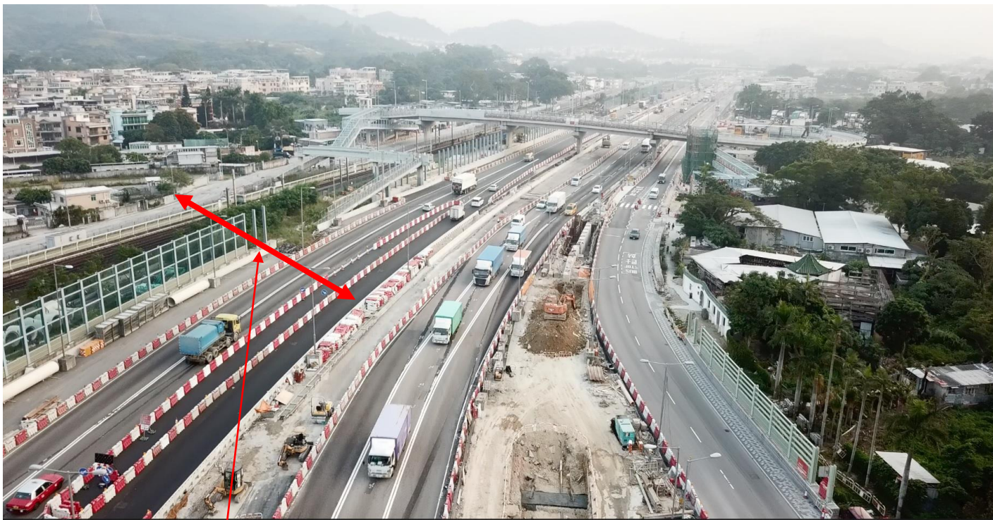
Photo 1: Site photo showing the construction works area and monitoring location (Date: 8 December 2017)
