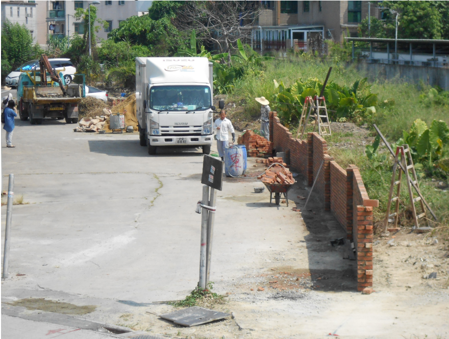
Photo 2: Construction of a brick wall with a stockpile of sands observed near the monitoring station SR77 (Date: 17 October 2014)
