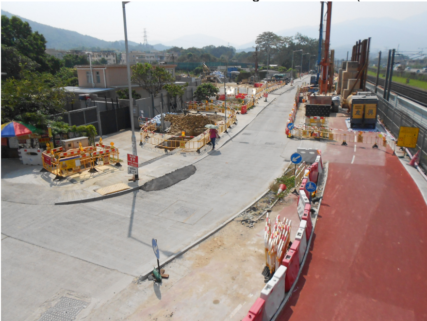
Photo 3: Excavation works under another contractor for Highway's Department observed near the monitoring station SR77 (Date: 17 October 2014)
