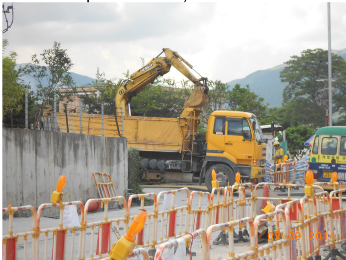
Photo 1: Handling of spoils observed within close proximity of SR77 (Date: 2 September 2014)
